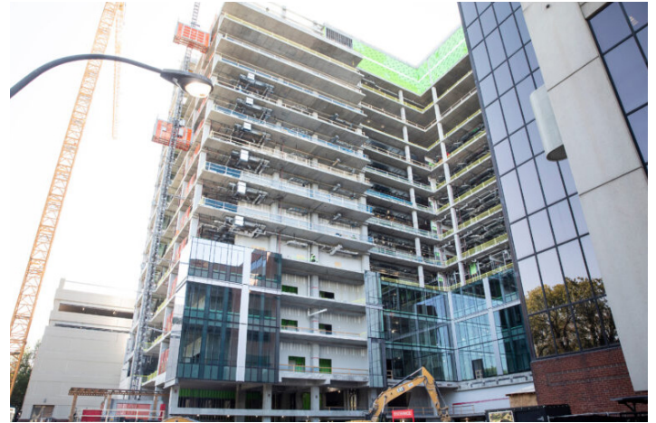
Construction of the new tower is taking place amid the daily hustle and bustle of Vanderbilt University Medical Center's campus on 21st Avenue in Nashville. This picture captures progress as of early October 2024. (photo by Susan Urmy)
